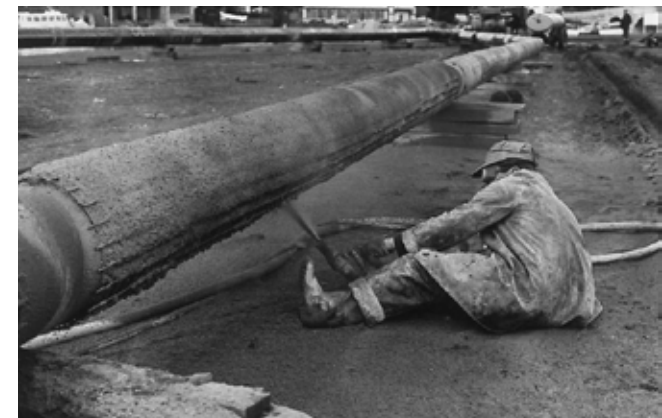
1963 - A workman applies a concrete coating to one of the pipes from Fawley to London to protect them from any damage which may occur on the river bed.
